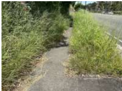
Unchecked vegetation can block sidewalks and decrease visibility
