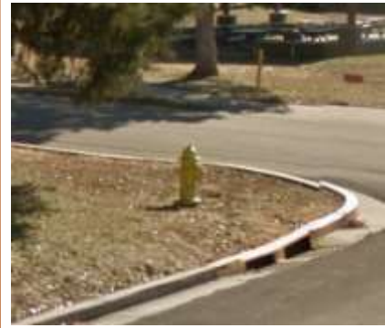
Fire hydrants provide needed water to fight fires and allow water lines to be flushed to keep the water clean. They can also be tested to check the water pressure and flow in the area.
