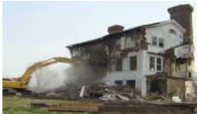
Demolishing houses can make room for redevelopment and remove nuisances. But demolition also removes older, historic buildings and can create voids.
