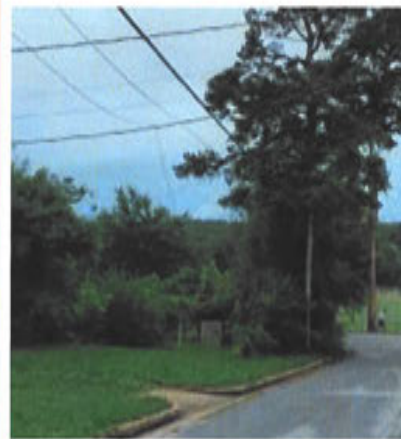
Utility lines and poles operated by franchise utilities for phone, cable, ect. have been poorly maintained in the neighborhood
