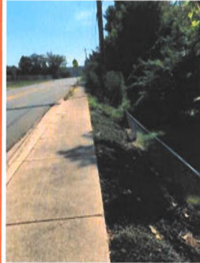
The sidewalk adjacent to 18th Street is directly adjacent to the road, narrow, and is adjacent to a steep slope with no guard railing
